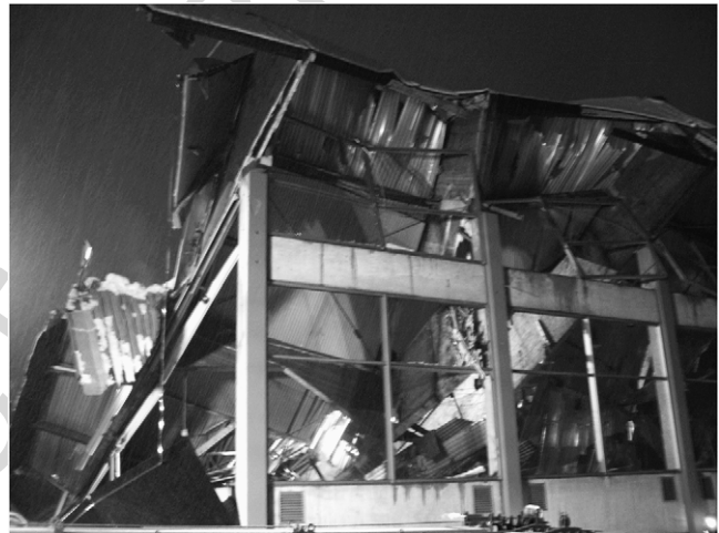
Fig. 5. Partial view of the collapsed roof structure.
