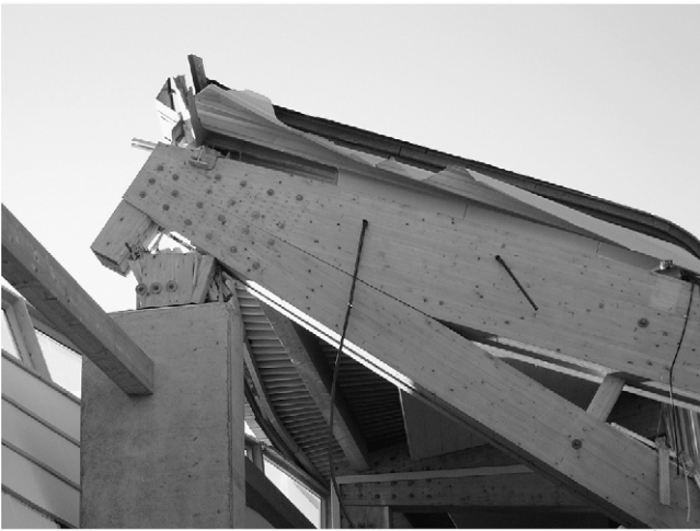
Fig. 2. Corner connection with concealed steel plates, connecting the timber parts through bolts (visible) and dowels (not visible).
