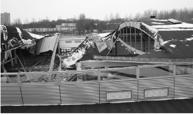
Fig. 1. The Siemens arena roof structure after the collapse of two trusses. An intact truss can be seen on the right.
