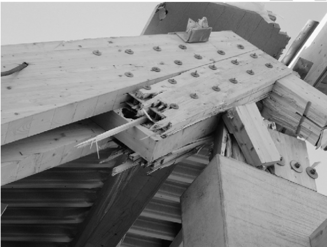
Fig. 3. Rupture at the critical cross-section in the corner connection. Note the dowels and steel plates.
