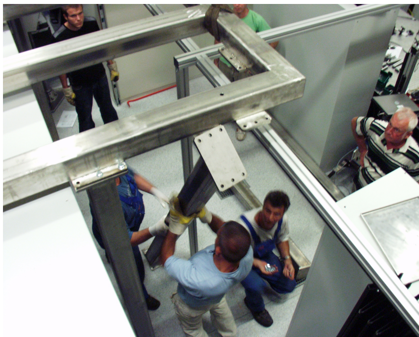
Figure A.4: To stabilize the bridge above the laser huge steel pillars are needed.
