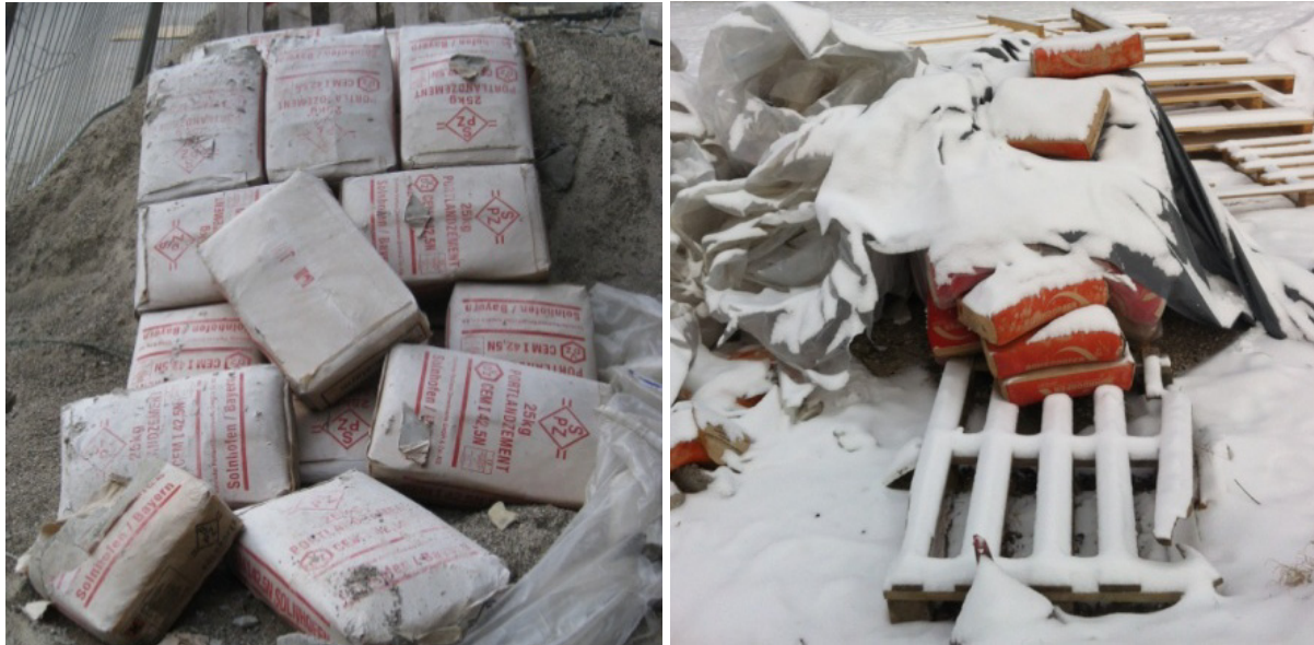
Figure 1: Photos of cement bags on a construction site, illustrating inappropriate storage conditions in summer ( left ) and winter ( right )
