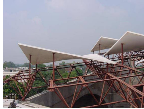
Fig. 8.0 Hyperbolic Paraboloid Shell: 5.0 M x 5.0 M 75 mm th. Light Weight Sand-which panel construction.
