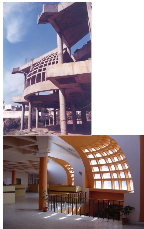
Fig. 5.0 Southern face Solar Shells: In construction and Interior distribution of daylight (winter) when completed.
