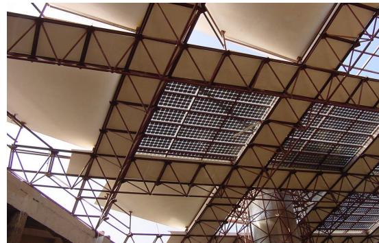
Fig. 9.0 Atrium roof BIPV: Integration of PV Systems through Glass to Glass Sand-which panels.
