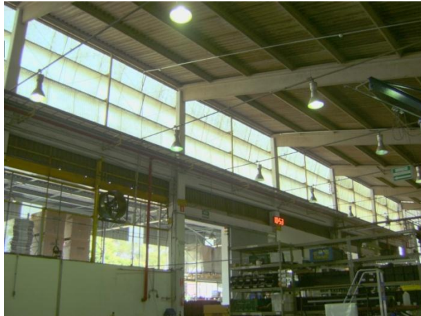
Figure 2: HDR image in Industry A - lack of integration between lighting systems.
