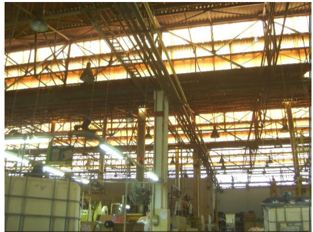
Figure 4: HDR image in Industry B - lack of maintenance of daylight capturing systems.
