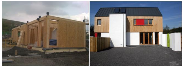
Figure 4: A Low Carbon House constructed from indigenous timber using the Ti Inos system.
