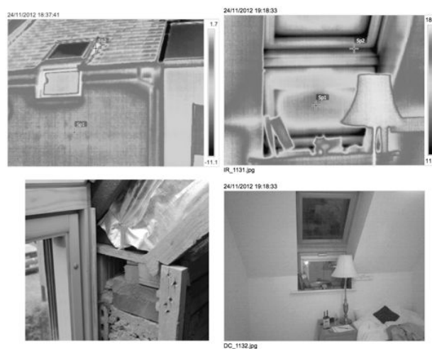
Figure 5: Thermal weaknesses at window openings
