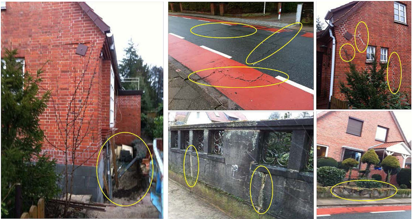
Fig. 18. Pictures of the area of the bigger subsidence bowl in Lueneburg, “Ochtmisser Kirchsteig,” which has been detected using DSI (i.e., the region surrounding point A marked in Fig. 15).
