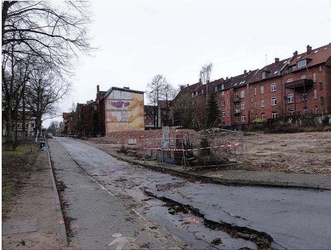
Fig. 19. Picture of the area of the smaller subsidence bowl in Lueneburg, "Frommstrasse," which has been detected using DSI (i.e., the region surrounding point B marked in Fig. 15).
