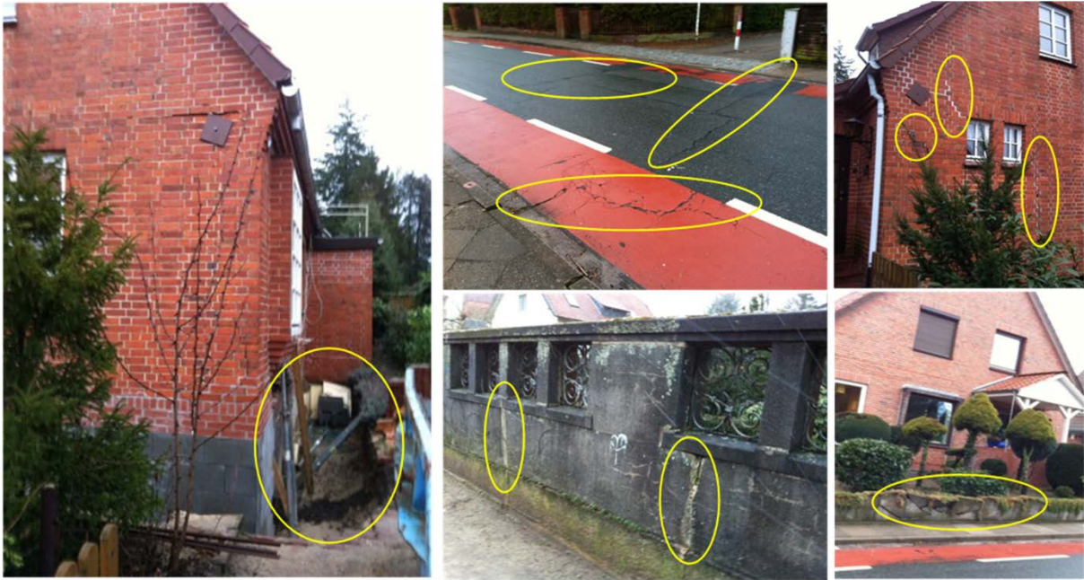
Figure 50: Pictures of the area of the bigger subsidence bowl in Lueneburg, ‘Ochtmisser Kirchsteig’, which has been detected using DSI (i.e. region surrounding point A marked in Figure 47).
