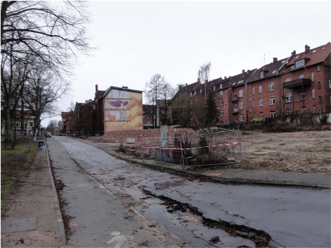
Figure 51: Picture of the area of the smaller subsidence bowl in Lueneburg, ‘Frommestrasse’, which has been detected using DSI (i.e. region surrounding point B marked in Figure 47).
