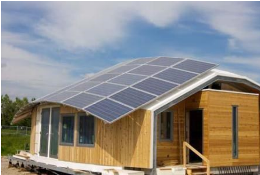
Figure 2-7: Building Integrated Photovoltaic System in Canada by Schletter and SkyFire with “turtle” roof shape [2-10]
