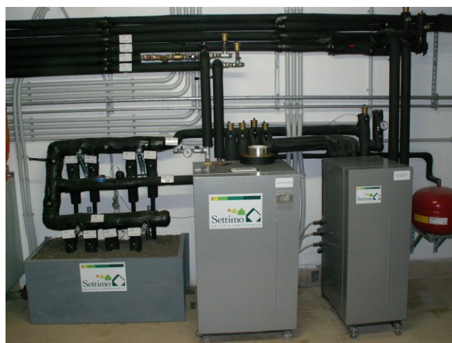
Figure 2-10: A GSHP, centre, left connections with two boreholes with two tubes each, right the free cooling unit
