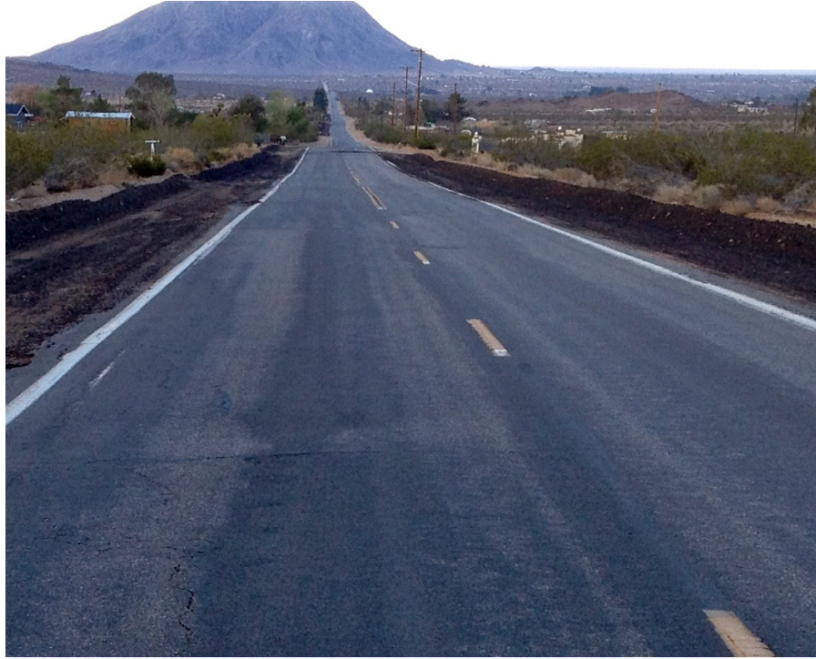
Figure 30: Right-lateral offset of Linn Road, Landers CA 92284, USA caused by the 1992 Landers earthquake. 23 years after the earthquake the offset is still visible. The picture was taken on July 5, 2015 looking eastward at 34.2954^\circ , -116.4554^\circ .
