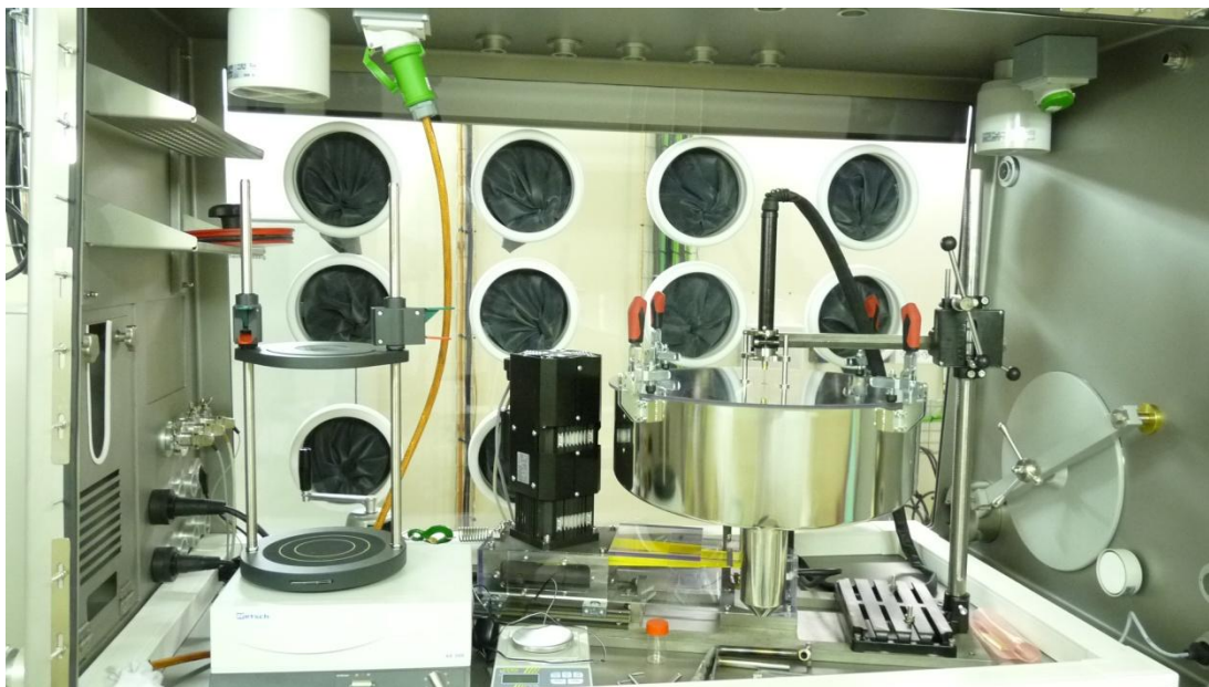
Figure 3-9 Inside view of the atomizer glovebox before hot commissioning, showing the atomizing unit, sieving machine for powder granulometry, and weighing scales.
