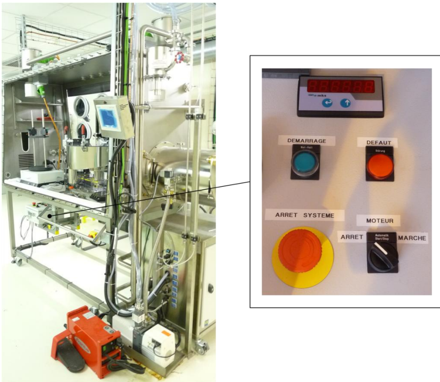
Figure 3-41 Extricable VFD control panel, situated underneath the atomizer glovebox bottom plate.
