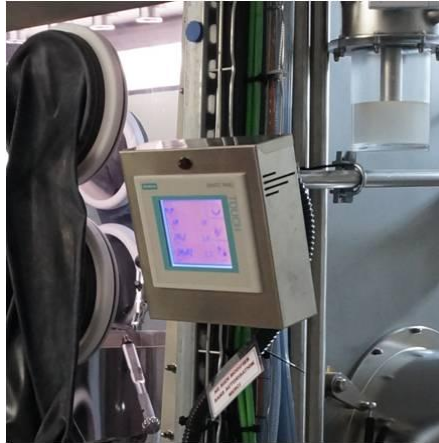
Figure 3-17 Control panel of the gas purifier.
