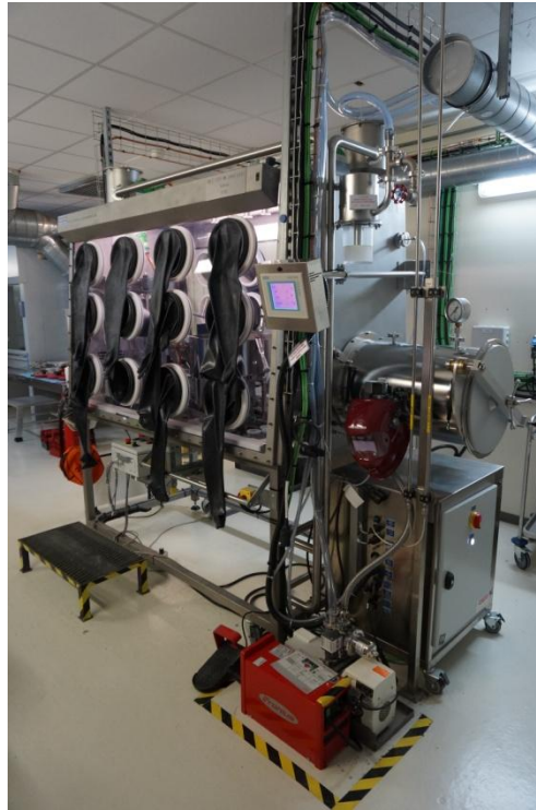
Figure 3-6 Atomizer infrastructure during hot operation in the UMo laboratory.
