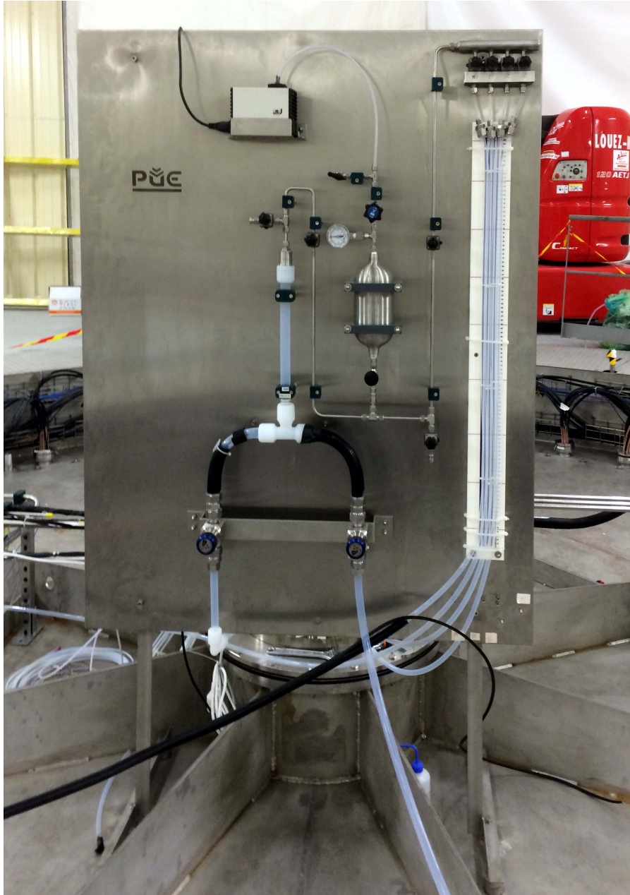
Figure 4.16: Cross reference system (XRS) and Loris Tube panel after installation in the near detector laboratory. In the middle there is a buffer volume connected to a vacuum pump. The buffer volume can be connected either to the inverted syphon, called Loris Tube, (left side) or to the XRS (right side). The XRS consists of four tubes, which are connected to each of the four detector volumes, respectively. If the pressure is decreased in the distributor at the top, the liquid level can be sucked up into the transparent tubing on the panel and the levels can be compared relative to each other.
