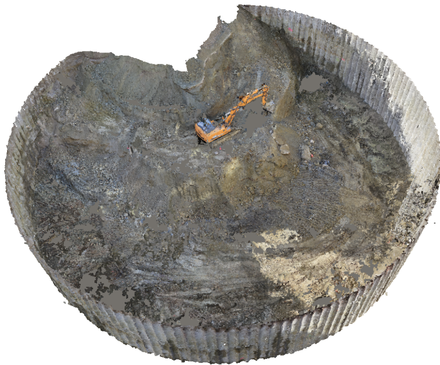
Figure 8.6: Point cloud of the underground parking garage excavation site. Lifting soil out of the pit slowed down the excavation progress.
