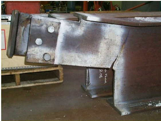
(a) Crack in steel structure [Mann, 2011]
