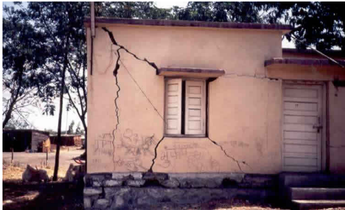
(b) In-plane wall cracking due to Killari earthquake in 1993 [WHE, 2016]
