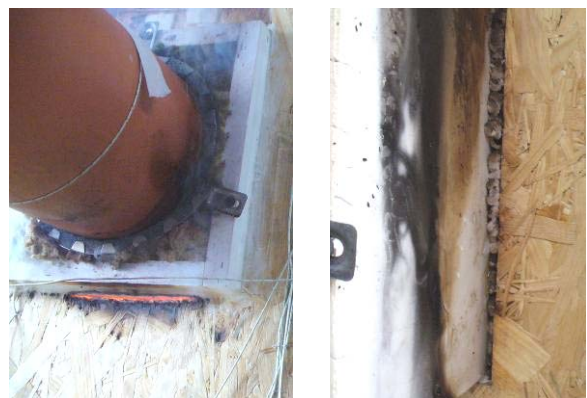
Figure 10: failure in sealed penetration junction (left); insufficient sealing with gypsum putty (right)
