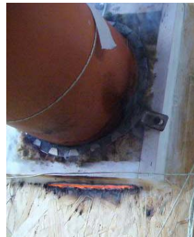
Figure 7. Failure in sealed penetration junction
