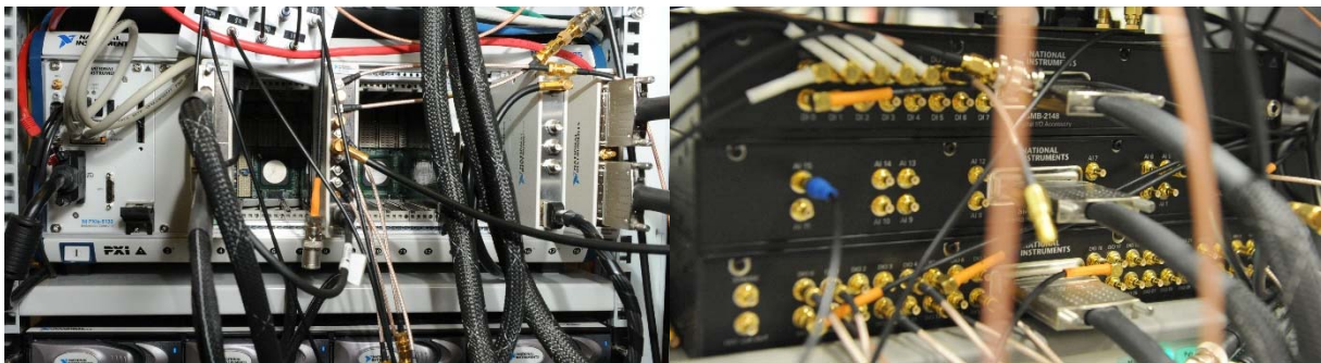
Figure 4.2: Integration of FPGAs into experimental setup. The possibility to code hardware functions directly into an FPGA reduces number of devices and required interconnects. The FPGAs in the PXI-express rack are shown on the left side. Cables lead to breakout boxes where the individual signals are picked up.
