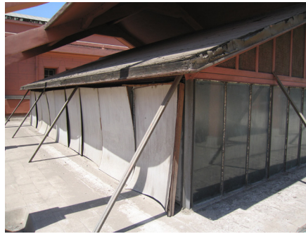
Figure 5.34 (left) The skylights on the West Wing. All existing skylights over the West Wing and East Wing have the same construction.
