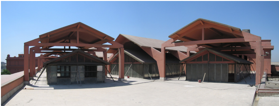
Figure 5.36 The skylights over R15, R14 and R9 on the east and North Wing.
