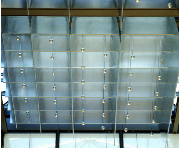
Figure 1.43 Close up photos for the daylight grid louvre ceiling. Art Museum Wolfsburg, Germany. (with permission of Bartenbach GmbH).
