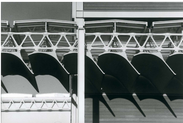
Figure 1.31 External view from the Menil Collection galleries, Houston, USA. A part of the roof and ceiling construction was used externally as shading device. We can see carefully from this photo the construction of the glass roof and the ceiling 'leaves'. ( http://www.rpbw.com/project/25/the-menil-collection/# ).
