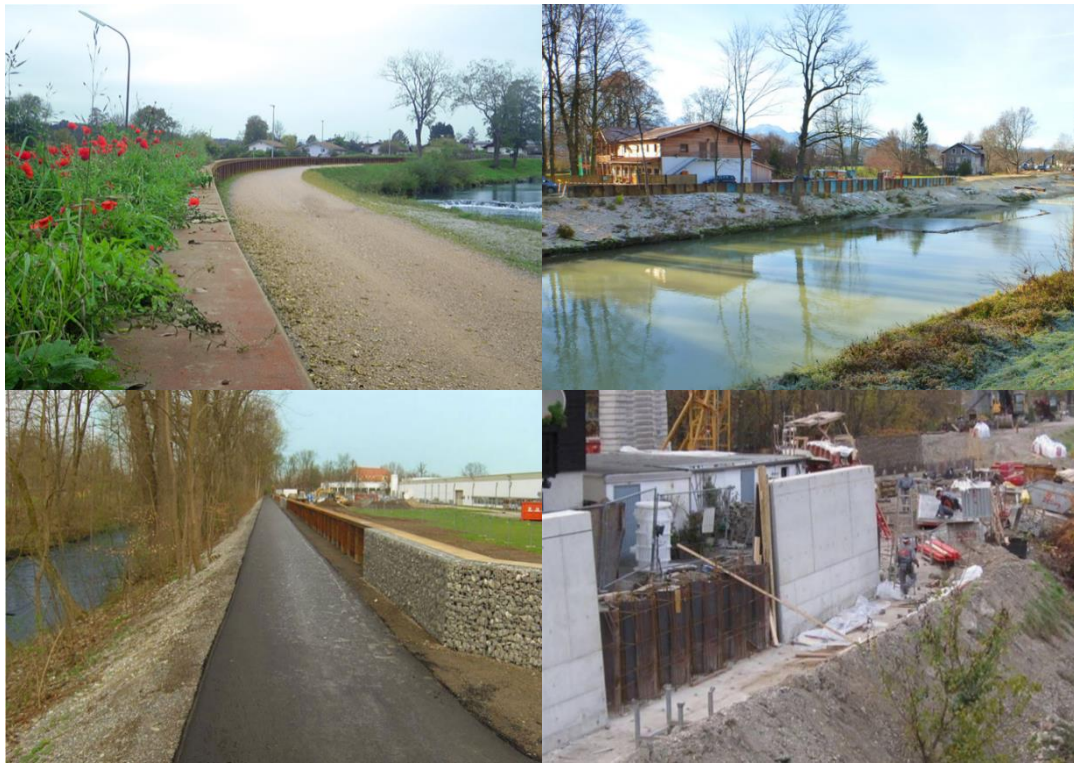
Figure 5-3. Recent construction efforts to increase flood protection in Rosenheim. Top row: Dike fortification using sheet pile walls. Bottom row: flood walls placed on dikes. Photographs from (Wasserwirtschaftsamt Rosenheim, 2017).
