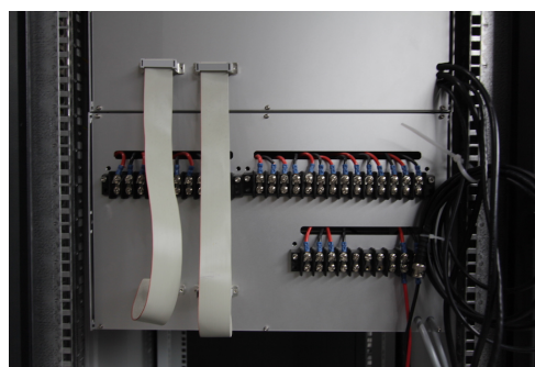
(b) View of the connection terminals where the coils have to be connected.
