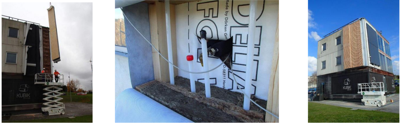
Figure.5: The demonstrator at the Kubik building, based on the installation of the modules, fitting the services and final finishing.
