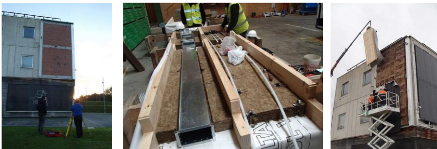
Figure. 1: BERTIM project is based on the accurate data acquisition, digital design with the help of RenoBIM, CNC manufacturing, assembly and rapid installation.
