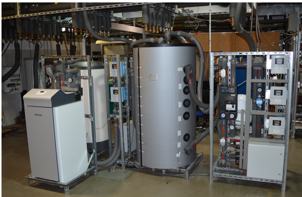
Figure 2. The three modules and the heat pump installation in the lab.
