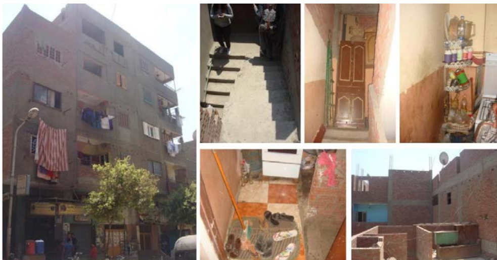
Fig. 2. Status quo of selected case study building (Photo credit: Dr. Wafaa Nadim, 2016)
