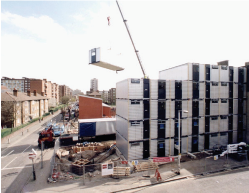
Fig. E.1: Installation of modular units at Murray Grove, Hackney, London (Yorkon)
