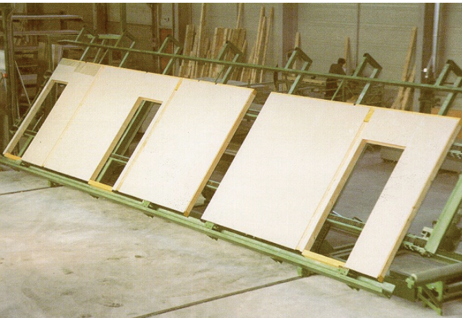
Fig. H.9: Tilting station
