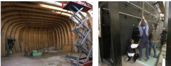
Fig. F.24: interior view of the wood structure and construction of the facade-elements
