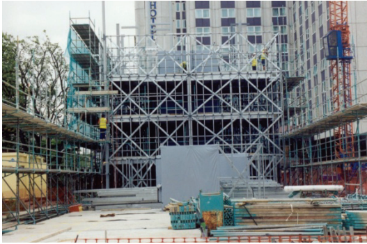
Fig. E.13: Load-bearing braced walls and stacked bathroom modules in the project shown in Fig. E.2
