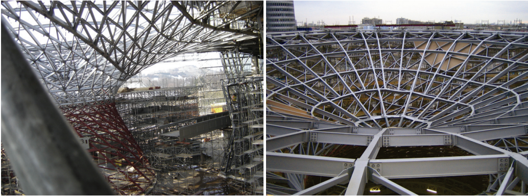
Fig. D.7: Coophimmelb(l)au Tornado, view of the prefabricated steel structure on site
