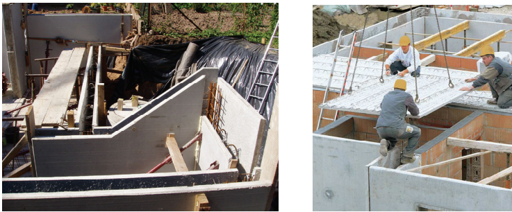
Fig. C.4: Rationalisation through the use of prefabricated components (e.g. hollow reinforced concrete walls and semi precast elements)
