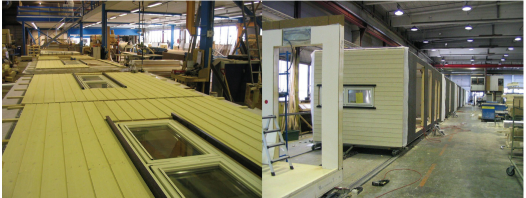
Fig. E.2: Modular housing construction quickly developed with the rise of industrialised production, and continues to thrive today. Possibilities for design variations tend to be very limited even in contemporary production settings.
