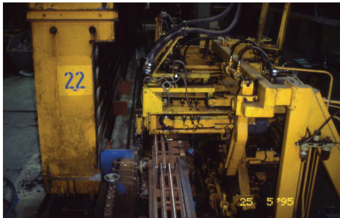
Fig. B.11: automated reinforcement (horizontal) station
