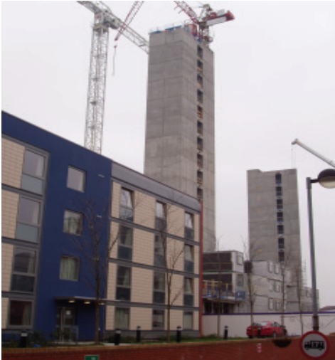
Fig. E.5: High-rise modular building in west London using a concrete core for stability (Caledonian Building Systems)
