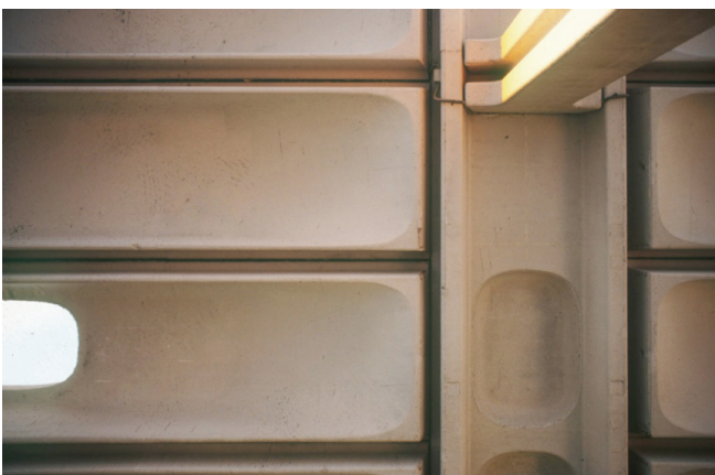
Fig. B.4: Underside view of floor with Isocell U70, Turate (Matthias Bräm)
