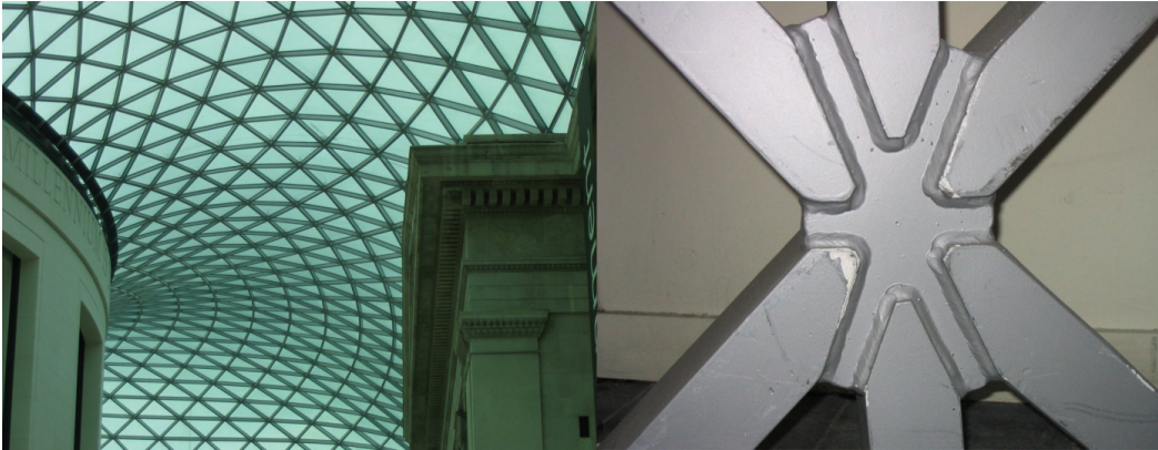
Fig. E.4: Parametrically varied members of the grid shell covering the British Museum courtyard. The members were welded on an automated welding robot to CNC cut node plates (right)
