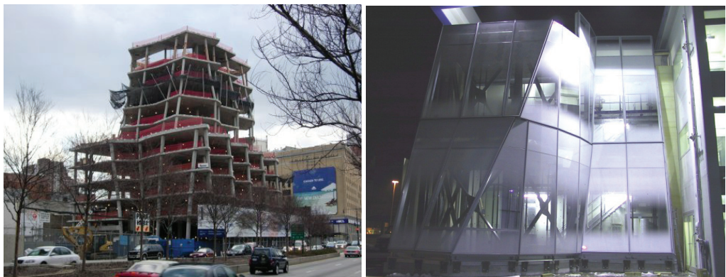
Fig. D.9: IAC building in New York by Gehry Associates, 2007. Structure installation and envelope installation.
