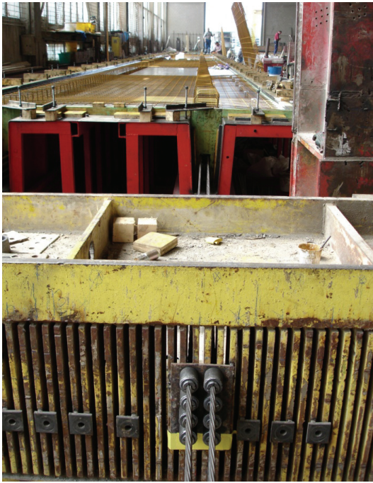
Fig. G.11: Prestressing strands in a stressed bed (Element AG)
