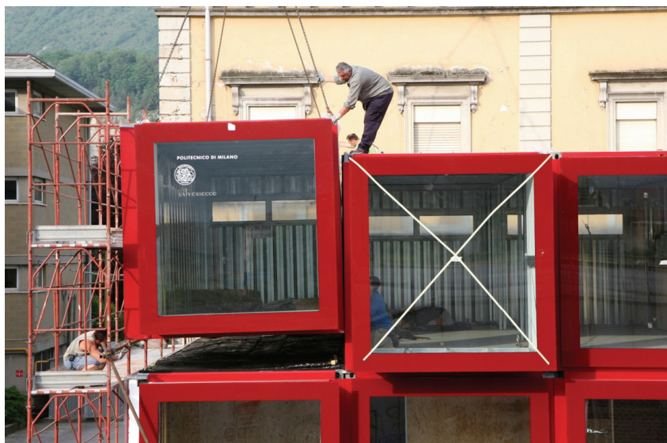
Fig. C.20: Research Campus Point in Lecco: Construction phase of the building (SANDRO BACCHI, STUDIO ARDEA, 2007)
