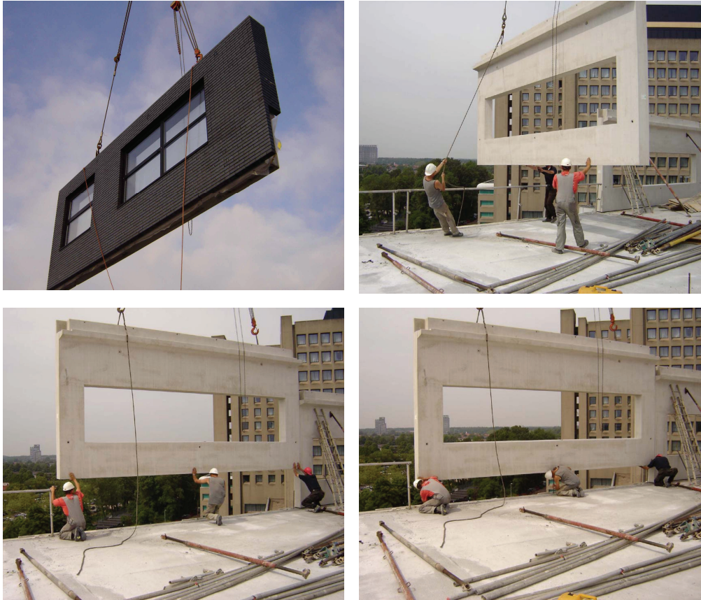
Fig. G.4: Getting the façade unit in the right position. As soon as the unit is kept just above the starter bars, the guard-rail is removed
