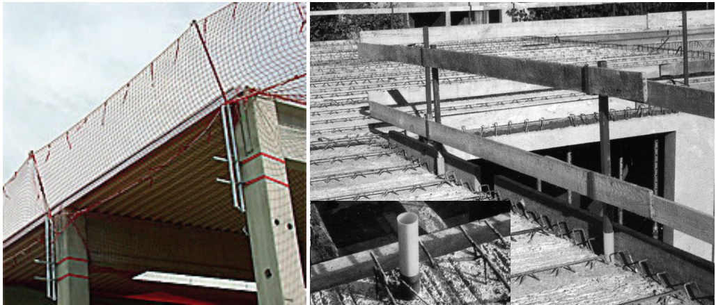
Fig. G.35: Safety fall protection following positioning of the prefabricated components (Leisering, 2006)
