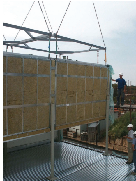
Fig. E.16: Installation of modules with recessed corners around SHS columns (OpenHouse AB)
