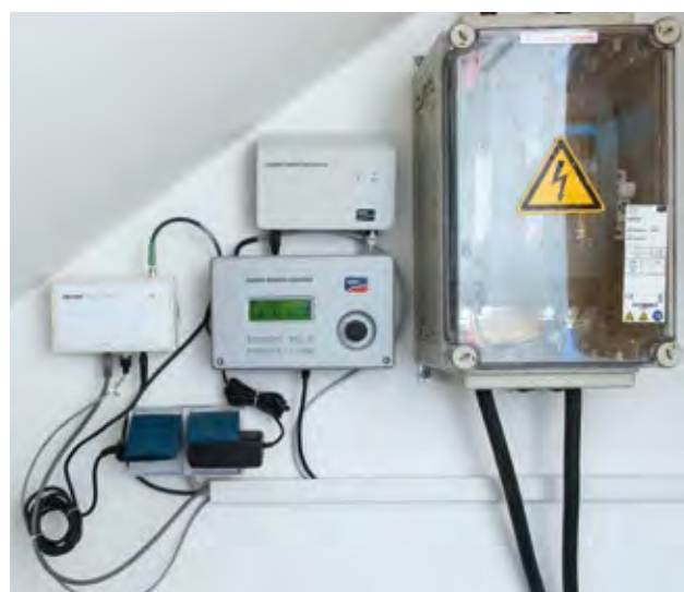
■ Components of the energy management system consisting of SMA Homemanager, SMA Remote Control, Stiebel Eltron ISG Plus and SMA battery fuse.
