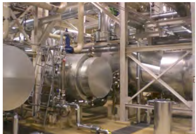
■ Geothermal Power Plant Sauerlach
