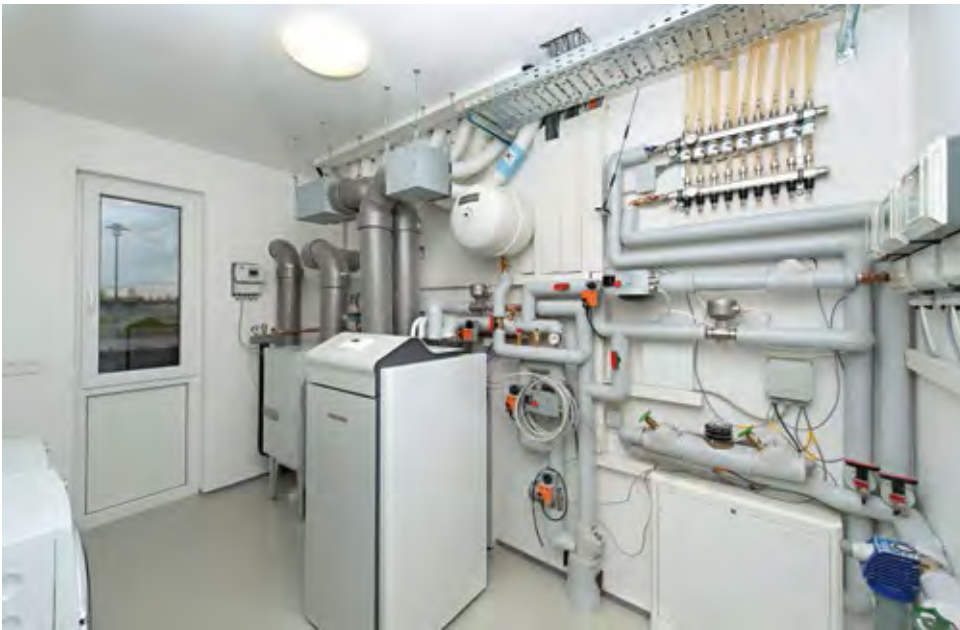
■ Heating system in the plant room of the Dynahaus consisting (from left to right) of the ventilation system, the air to water heat pump and the heat distribution system for the floor heating.
