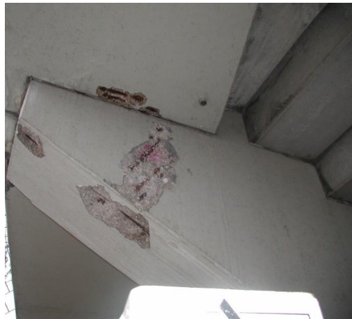
Figure 9: example of carbonation-induced corrosion (Olympic Arena, Munich) [62]
