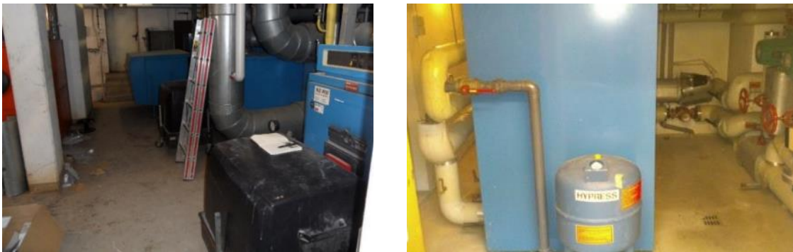
Figure 32: Central heating station with three gas boilers (building 1, left) and example of a substation with limited space (right)
