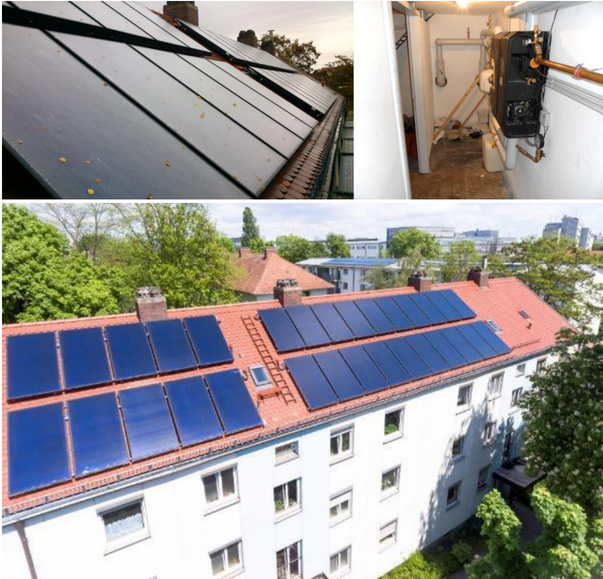
Figure 104: Building 2 – four parallel collector arrays (top left), solar station between primary solar circuit and district heating return pipe (top right) and full view (bottom)
