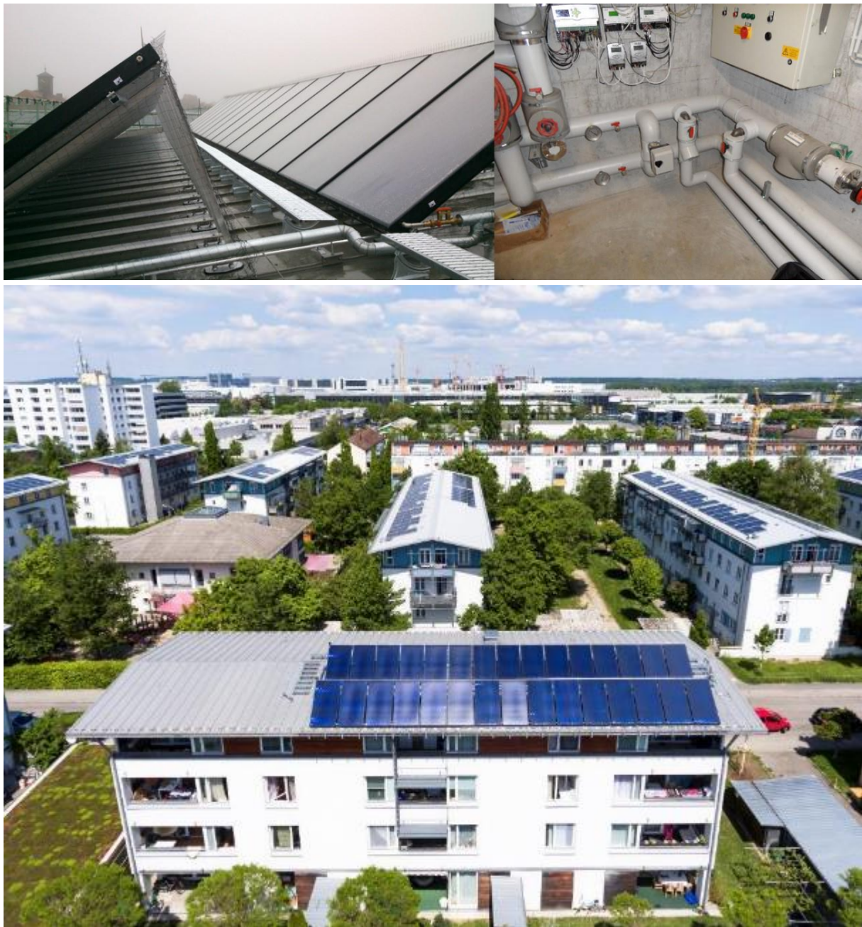
Figure 107: Building 4 – 40°-inclined collectors on the south roof (top left), controller, metrological equipment and feed-in components (top right) and full view (bottom)
