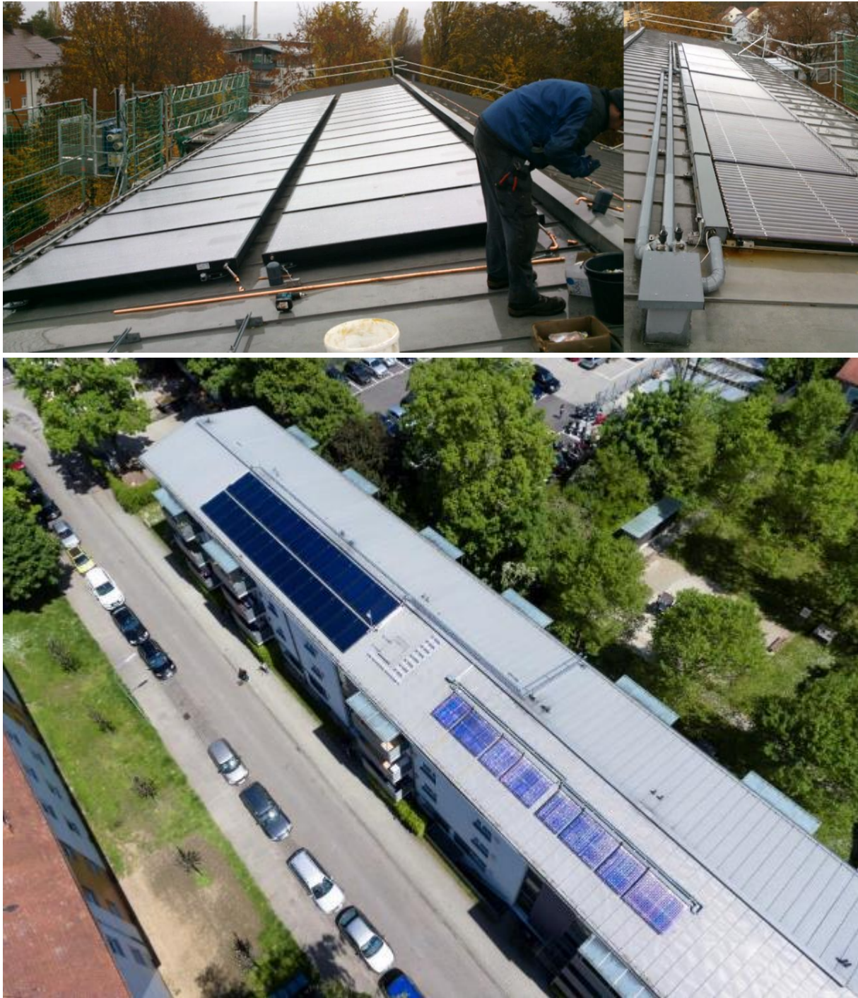
Figure 106: Building 3 – newly installed flat plate collectors (top left), existing evacuated tube collectors (top right) on west roof and full view (bottom)
