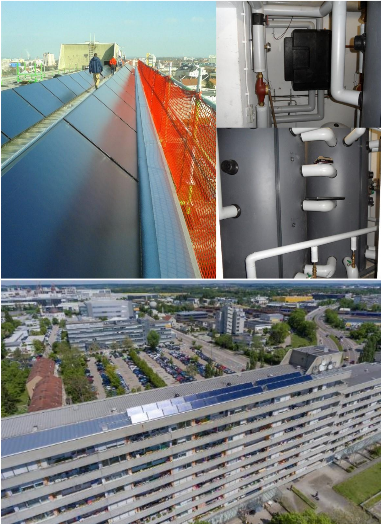
Figure 105: Building 1 – 40°-inclined collectors on flat roof (top left), solar station (top right), parallel connected buffers in the basement (mid right) and full view (bottom)
