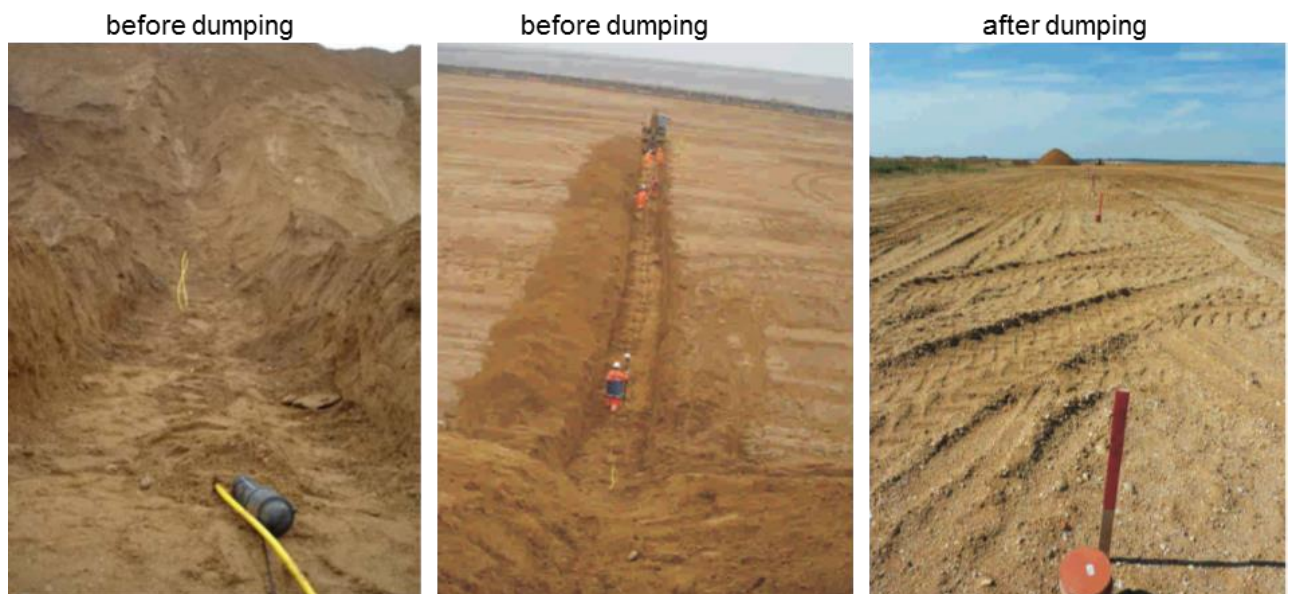
Figure A.12.2: Installation process of the hydrostatic measurement line, printed with permission from RWE Power AG
