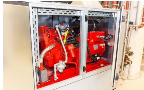
Fig. 9 CHP of Building 5
