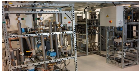
Fig. 8 Building 1 heat modules
