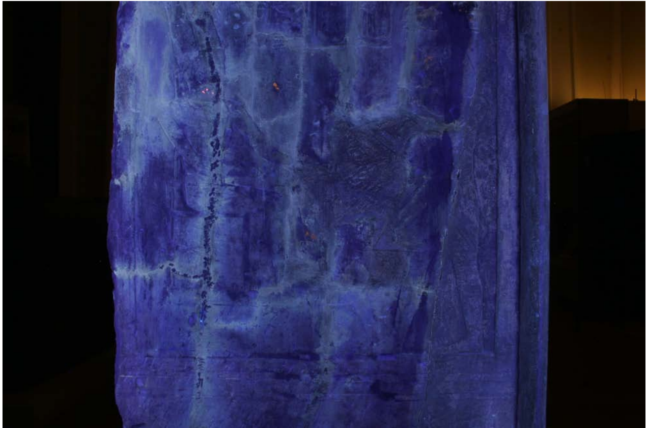
Figure 32 Scene lhs, UV image: 1969 retouched restoration mortar, shellac (orange spots)
