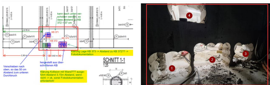
Figure 1.8: Error/inconsistency in the execution design; it was intended to have three openings (left) and drilled four incorrect openings (right) (Bollinger und Grohmann GmbH, 2022)
