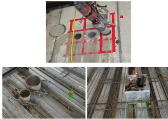
Figure 1.3: Example of execution of core drillings to make openings in concrete floor (top) and execution of pre-planned openings in concrete slabs avoid cutting (bottom) (Zamani, 2020)
