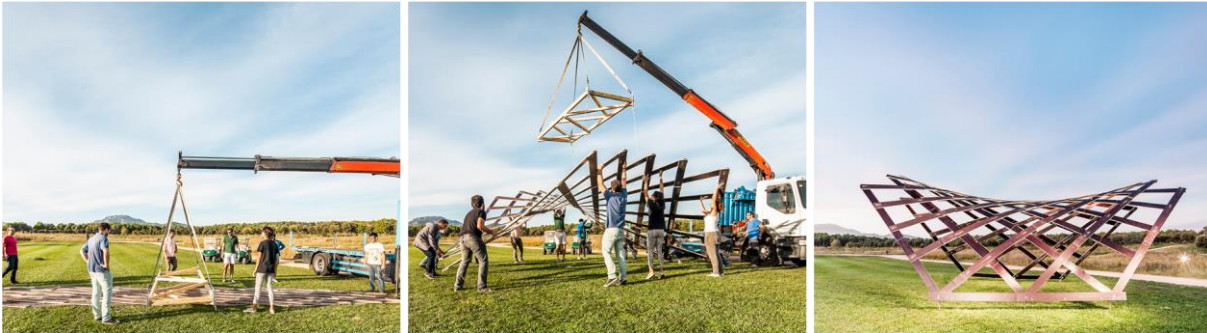
Figure 47 Erection of the “Neula”-pavilion in 2014 by Scientists of the UPC and CODA 1 (Photo: Andrés Flajszer)
