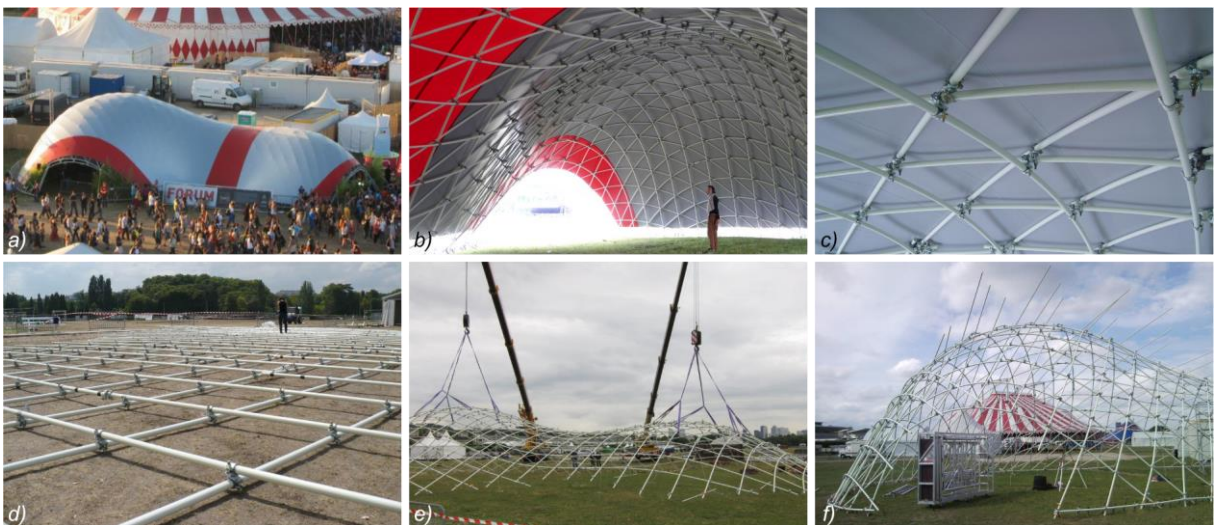
Figure 44 Gridshell at the Soliday Festival: a) View from outside, b) Inside view, c) Detail view d) Flat Assembly of the equilateral grid (two layers), e) Pull-up erection of the quadrilateral grid, f) Bracing (triangulation) at final geometry with third layer of GFRP tubes (TESS, 2011).
