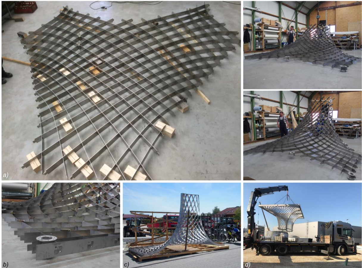
Figure 113 Erection the Hotel Intergroup canopy: a) Pull up of a grid segment, b) Assembly of edge components, c) Framed segment in final shape, d) Lift and transportation of the full steel structure
