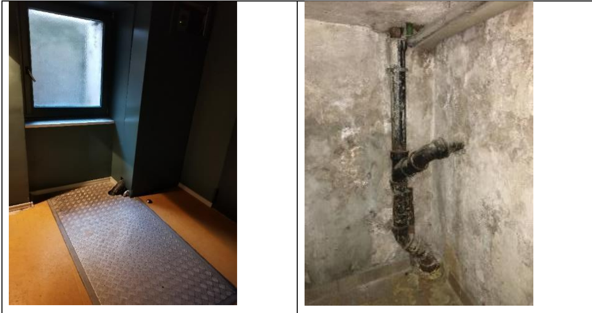
Photos showing the submersible sewage lifting pump that handle both waste and rainwater (relevant for KPIs B2.9 Backwater protection and B4.1 Separation of wastewater and rainwater)
