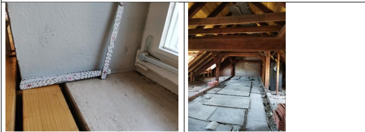
Photos showing the wall thickness and attic with floor insulation (partially damaged) (relevant to the KPI C1.2 Specific transmission heat loss of the building envelope)
