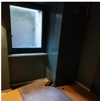
Figure 12: A submersible sewage lifting pump used in the basement of youth centre building to handle excessive rain events.
