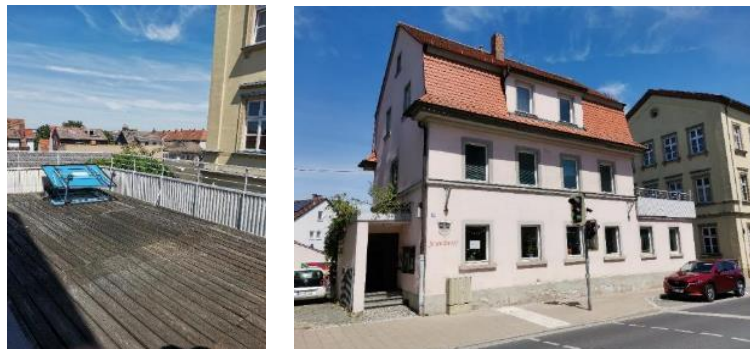
Figure 68: Images of the unusable balcony on the first floor and a view southern facing facade of the GAUstark Building
