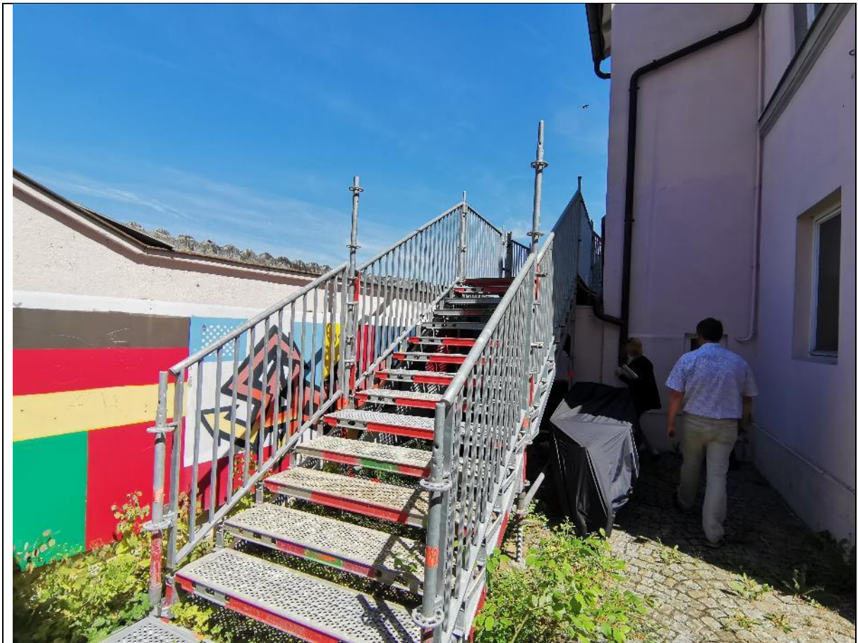
Emergency exist is an ad-hoc stating from the 1 st floor terrace and landing in cramped site (relevant for the KPIs B1.1 Availability of emergency response plan and evacuation routes for Hail, Snow and extreme precipitation events)
