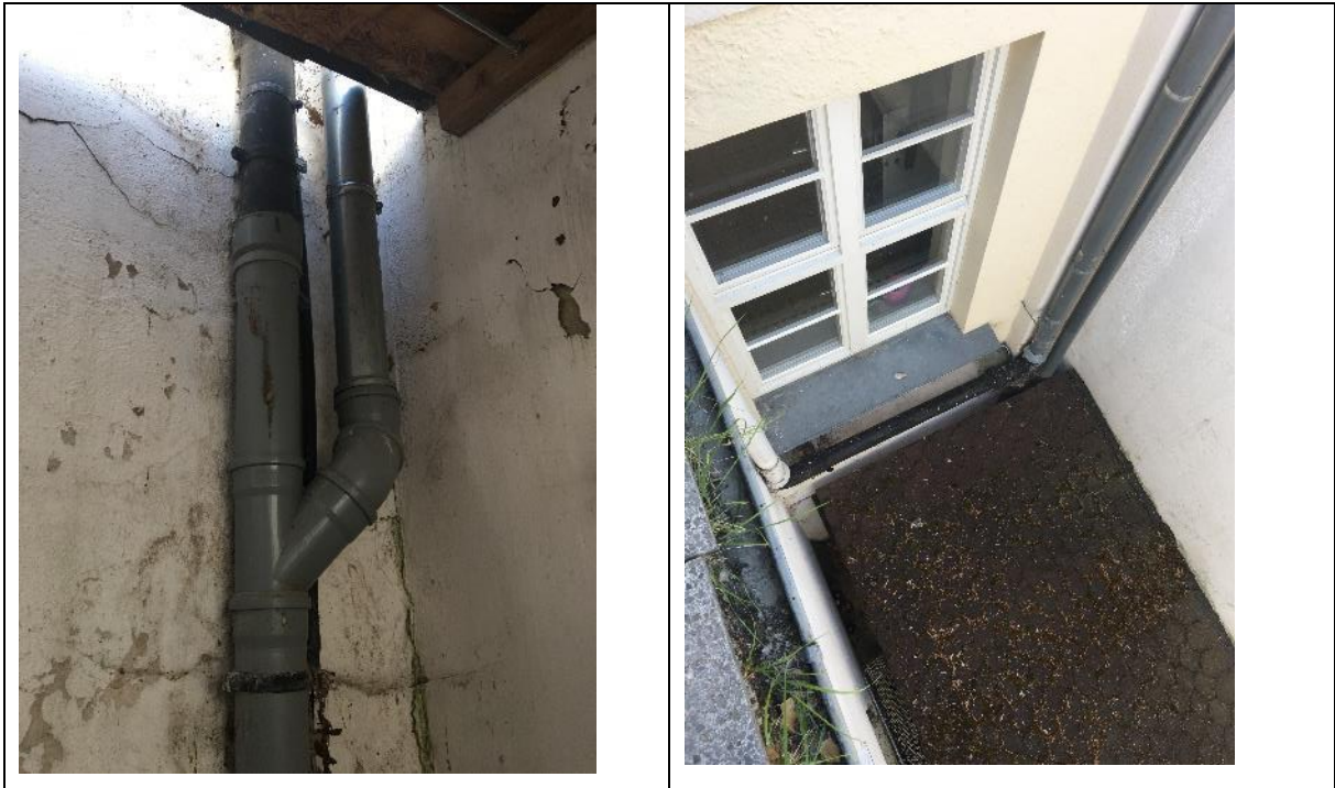
Photos showing the cramped and complicated paths of the rains and wastewater pipes as well as the unmaintained gutters (relevant for KPIs B5.2 Ease of maintenance/ retrofitting of Water, wastewater, and sanitation system and E5.1 Storm anchored external water supply and drainage systems)
