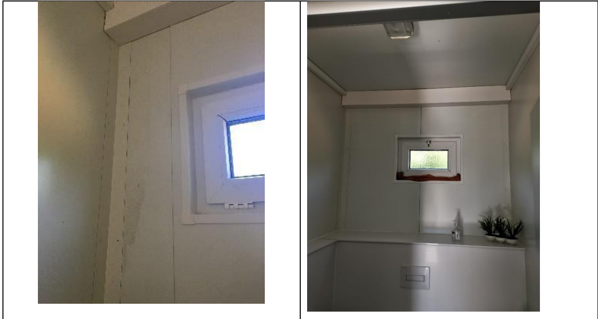
Photos showing signs of water and moisture damage in the toilets (relevant for the KPIs B2.1 Envelope moisture and rain protection and B2.6 Water Resistant Materials and finishes)
