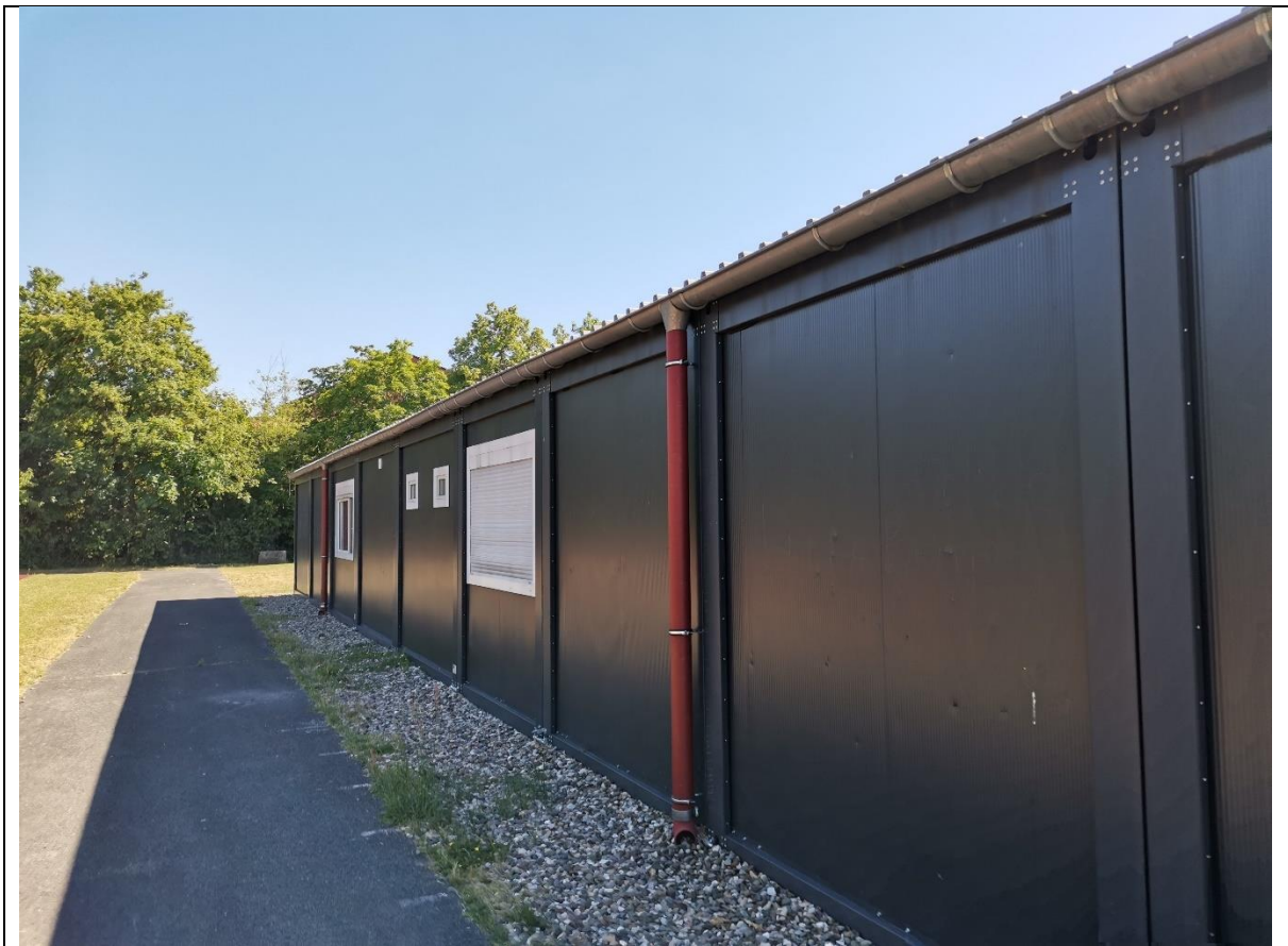
Photos showing the rainwater pipes (relevant for KPIs B2.9 Backwater protection and B4.1 Separation of wastewater and rainwater, (relevant for KPIs B5.2 Ease of maintenance/ retrofitting of Water, wastewater and sanitation system and E5.1 Storm anchored external water supply and drainage systems)
