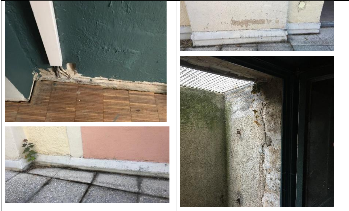
Photos showing the underground hall and part of the envelope impacted with water and moisture damage (relevant for the KPIs B2.1 Envelope moisture and rain protection and B2.6 Water Resistant Materials and finishes)
