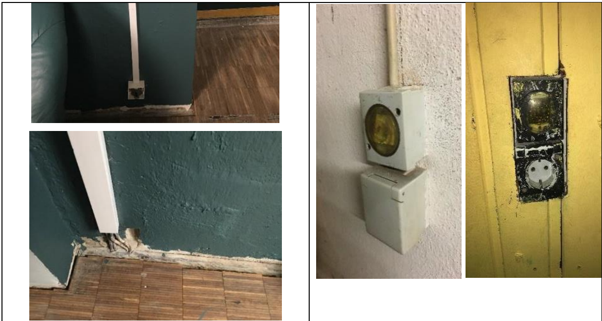
Not all electrical sockets in the basement retain their original water covers, some are not water resistance, and some cables are totally exposed (relevant for the KPI B1.5 Waterproof sockets and switches)
