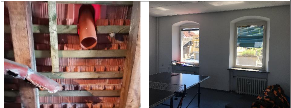
Lack of maintenance to the building technical and non-technical systems (relevant for KPIs B2.2 maintenance of building technical systems against extreme precipitation threat and C1.12 Maintenance of building technical systems against heatwave)
