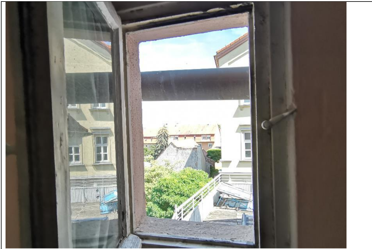
Photos showing the damaged and complicated paths of the rains and wastewater pips as well as the unmaintained gutters (relevant for KPIs B5.2 Ease of maintenance/ retrofitting of Water, wastewater, and sanitation system and E5.1 Storm anchored external water supply and drainage systems
