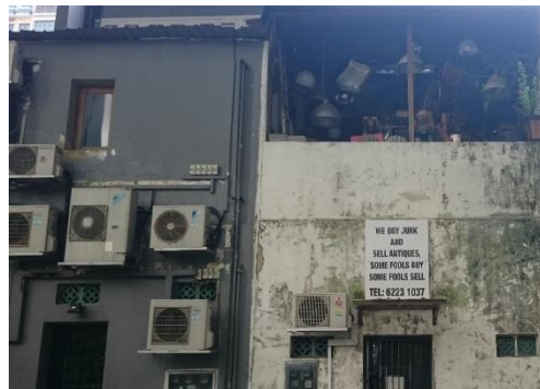
Figure 13: A collection of air-conditioning unites covering the shop fronts in Singapore
