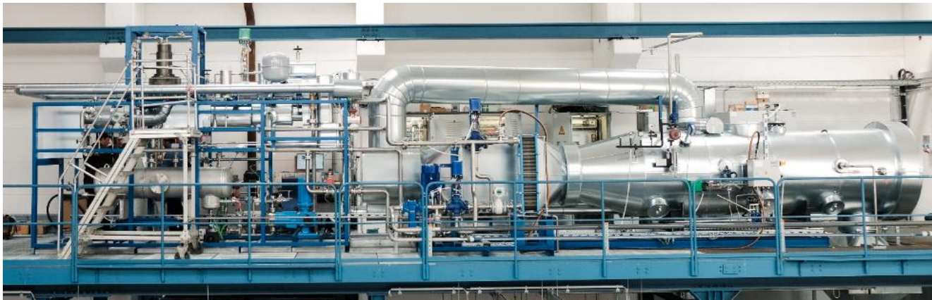
Figure 2. MicroRankine pilot plant at the sewage treatment plant in Nürnberg.
