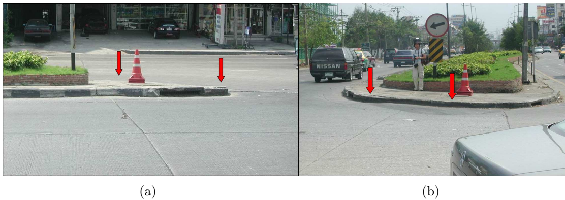
Figure 2.6: (a) and (b) show the unnatural and strongly uneven road surface of the two sides of a main road (passing from north to south of the study site) found in the study area.
