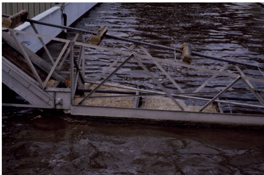
Figure 3: Scum harvester installed on the aeration tank of Australian WWTP-TH.
