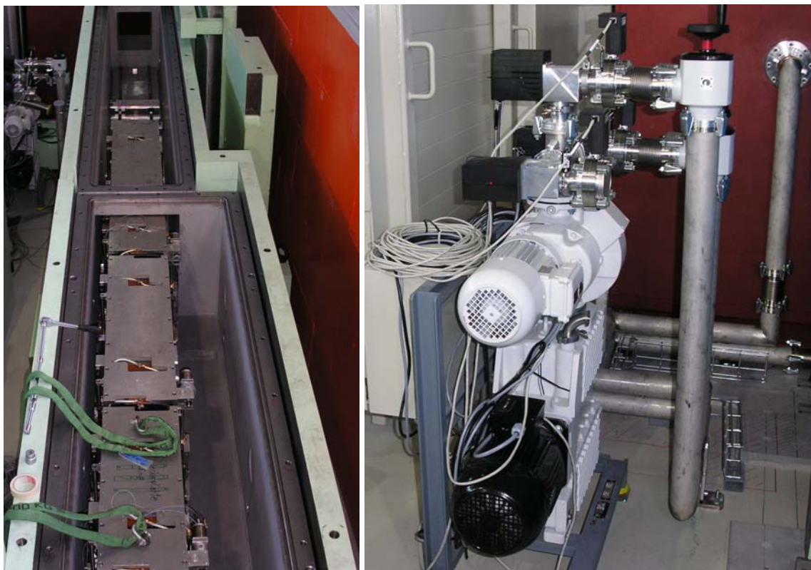
Figure AII.3 Photos of setting up the neutron guide elements (left) and the vacuum pump station (right).
