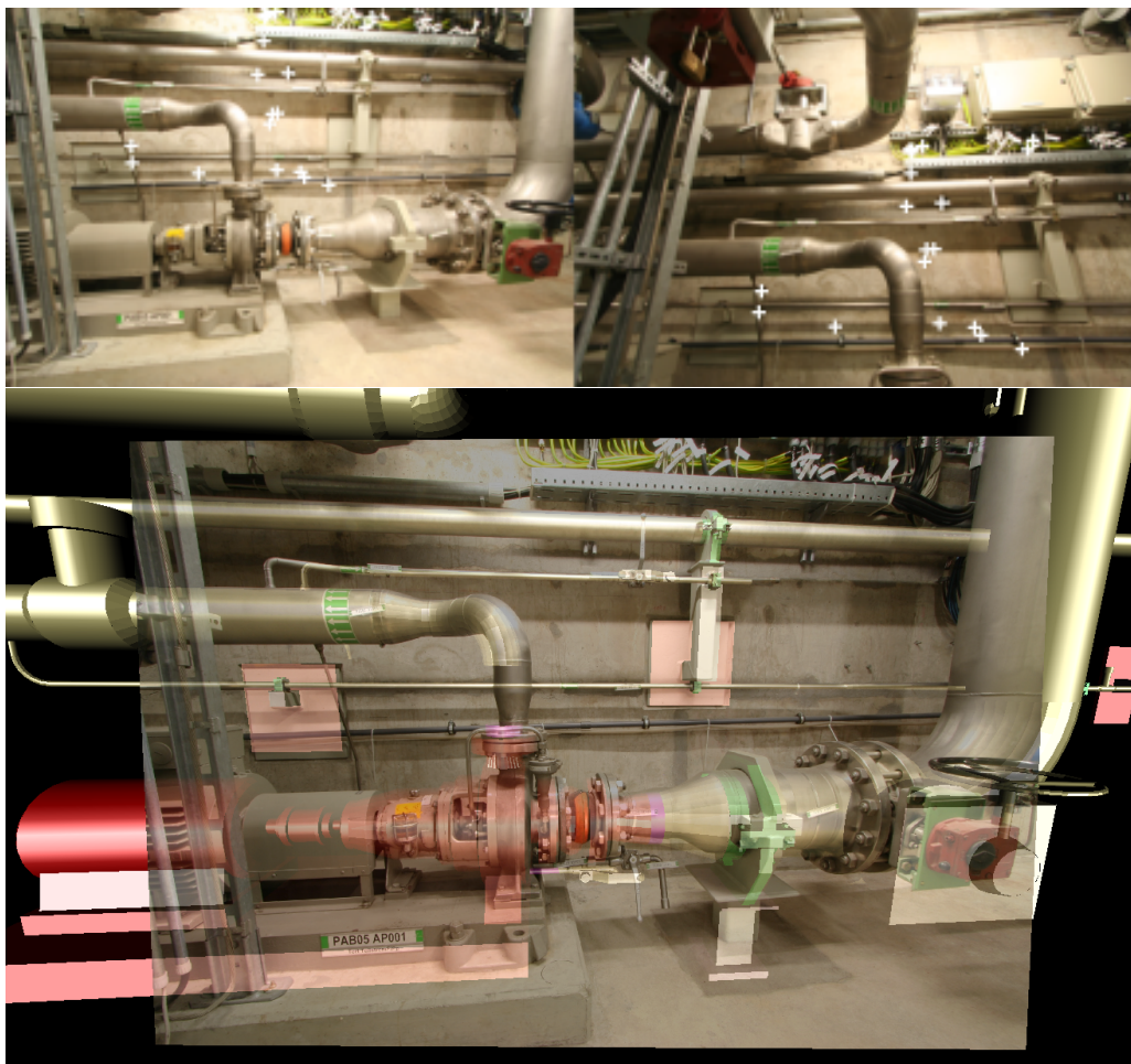
Figure E.1: Full Pose Estimation from a Single Keyframe Using Planes Matched features points are triangulated and planar structures are extracted and matched to the CAD model. The distance from the plane can be used to extend the relative pose to a full pose. Features matched to a CAD model plane are marked in white in the (top) images and the resulting augmentation is visible on the (bottom).
