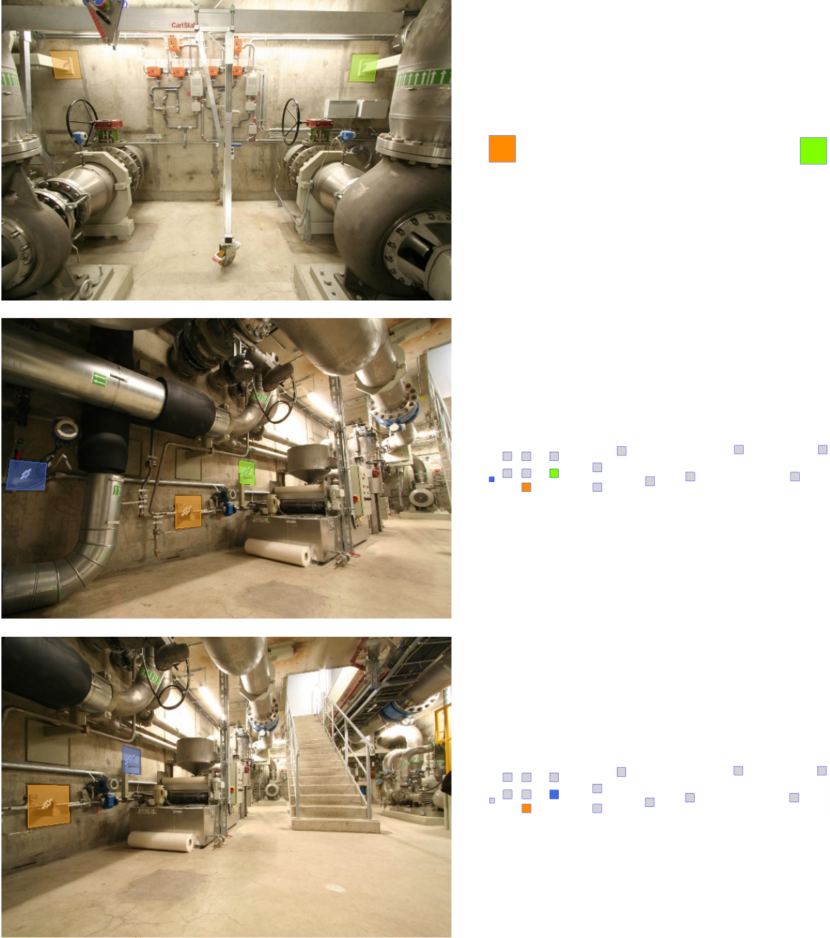
Figure 6.11: Anchor-Plates Matching Results 4 using images of a plant in operation. The algorithm used 3D information from the 4 walls ( Data-set 2 - Figure 6.3(b)) and segmentation provided from 6.2. It automatically detected the correct wall and matched to the correct structure.
