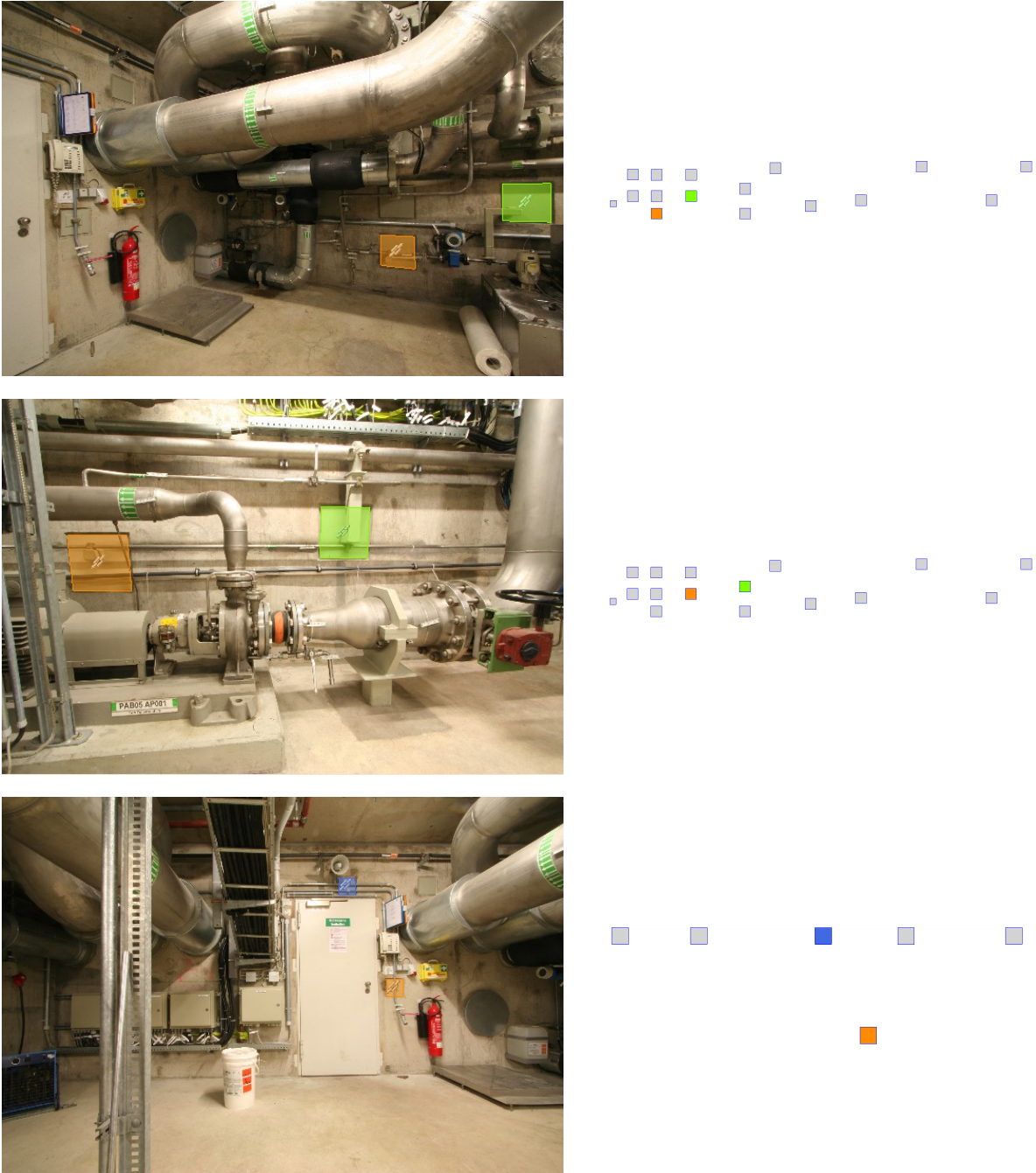
Figure 6.9: Anchor-Plates Matching Results 3 using images of a plant in operation. The algorithm used 3D information from the 4 walls ( Data-set 2 - Figure 6.3(b)) and segmentation provided from 6.2. It automatically detected the correct wall and matched to the correct structure.
