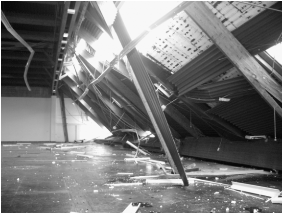
Fig. 17. Exhibition centre, failure of one main beam, development of hinges at supports of purlins [Photo: MPA BAU, TUM].
