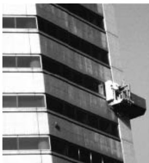
Horizontal-type facade robot, office building, Japan
