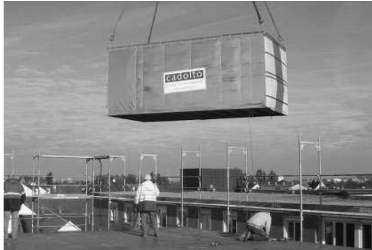
Figure 1-3: Conventional construction in practice: Supervision of unit installation process by four workers (3 operational floors, 1 ground floor) and one tower/mobile crane operator. The installation of the unit took 25 minutes. Cadolto construction site, Augsburg, Picture: Linner
