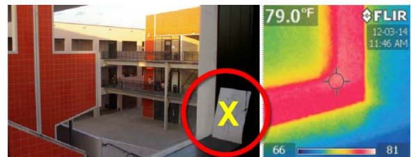
Figure 10: Right image: The FLIR infrared Image shows the outside surface temperature of the concrete precast of 98,8 F (37 C) and higher; while the air outside temperature is only 79 F (26 C) by a relative humidity of 78 % and 15 mph (24 km/h) wind pressure. Left image: The infrared image show the indoor surface temperature with 79 F (26 C) and higher of the noninsulated window frame area as a typical thermal bridge, while the air cooling supply in the Interior space is set by 54 F (12 C). Recorded on March, 12, 2012. Source: Author, 2012.
