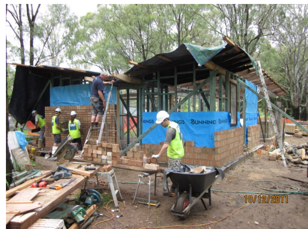
Figure 2. Work in progress showing the structural frame and masonry cladding at lower levels
