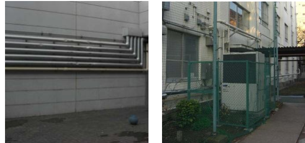
Figure 9: Problems of outdoor unit due to location.
