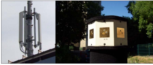
Figure 2. Transmit antenna (left) and receive antenna (right)
