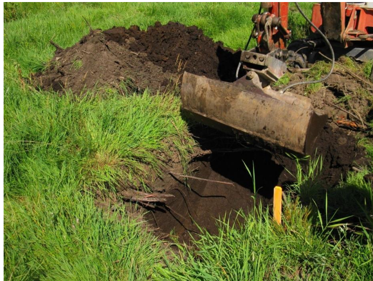
Figure 1.1. Excavation of organic soil in a road construction project located approximately 35 km northeast of Munich, Germany.
