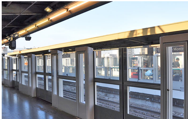
Figure 7.1: An installation of platform screen doors at a railway station.
