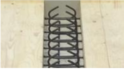
Figure 22: Element connection with glued-in reinforcement bars. To activate the force-fit, concrete is poured into the gap.
