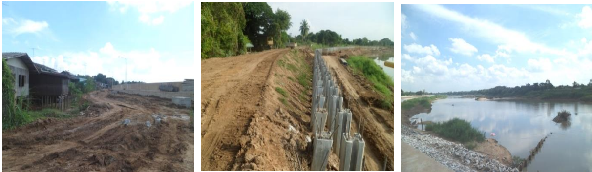
Figure 3.8 The public flood wall protection in Singburi province (Author)
