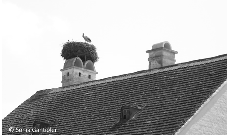
Figure 34: Artificial stork nest support, Rust (AT)
