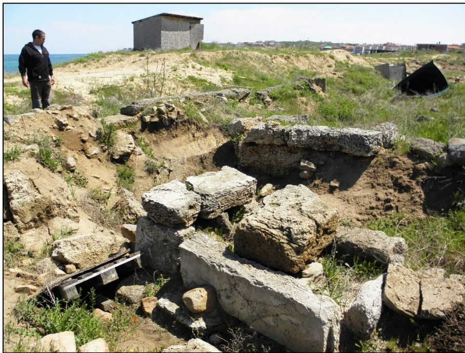
Fig. 34 Neglect after excavation has led to vandalism, erosion and partial loss at the necropolis of Roman Apollonia Pontica, Sozopol, Bulgaria
