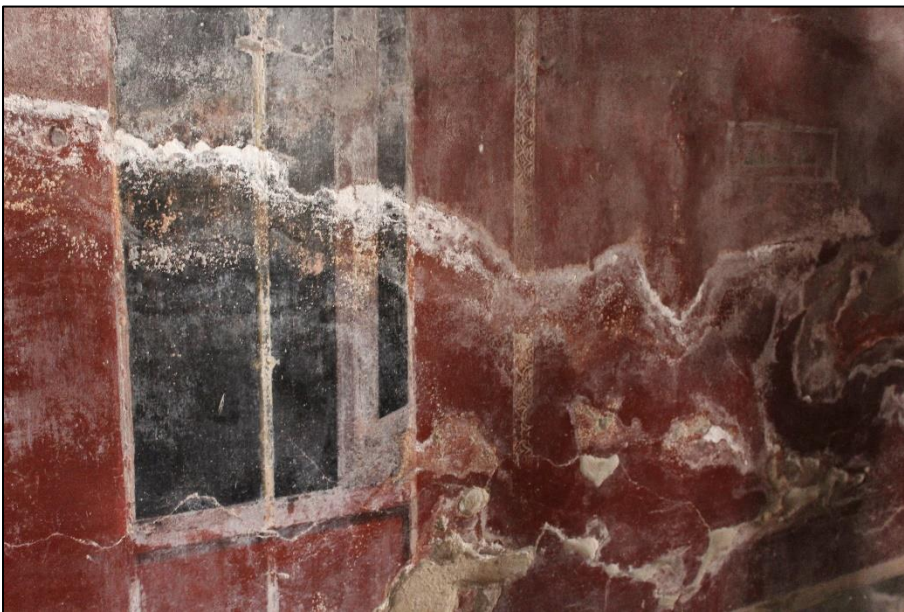
Fig. 19 Salt efflorescence on a wall painting at the WHS of Villa Poppaea, Oplontis, Italy because of the use of cement in the villa's restoration
