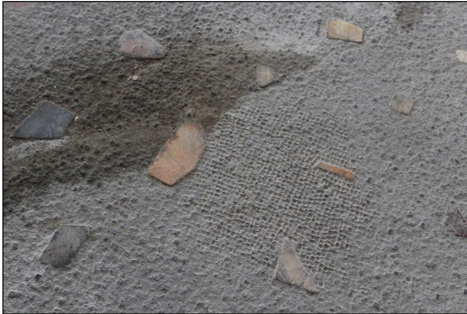
Fig. 17 Deteriorated floor mosaic at the site of Villa Arianna, Stabiae, Italy. Under the footsteps of visitors, fragile tesserae gradually disappear
