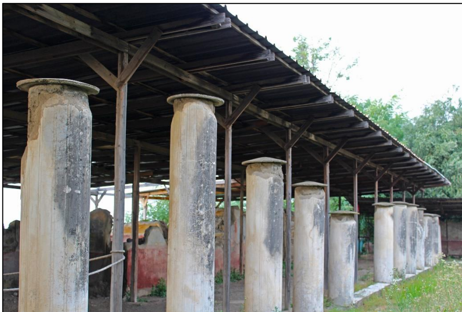
Fig. 10 A roof at the site of Villa Arianna, Stabiae, Italy failing to prevent wind-driven rain deterioration to the columns stored underneath it. Damage is clearly visible on all columns' ill-protected side
