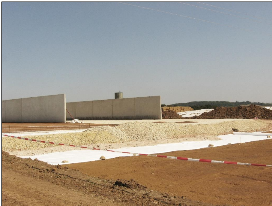
Fig. 30 Stratigraphy of the cover introduced over one section of the site of Ehingen am Ries – soil, geotextile, sand and gravel. A section of the power plant is under construction. Photo: J. Druckenmüller, KANT Archäologie GmbH. Courtesy of the Bayerisches Landesamt für Denkmalpflege
